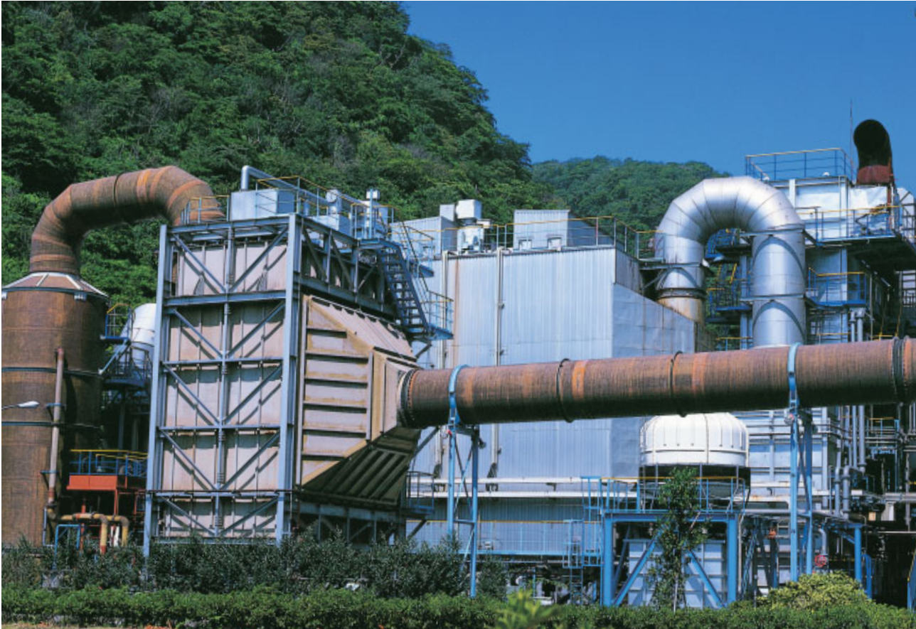
Incineration Plant, Nikko Environmental Services Co., Ltd.
