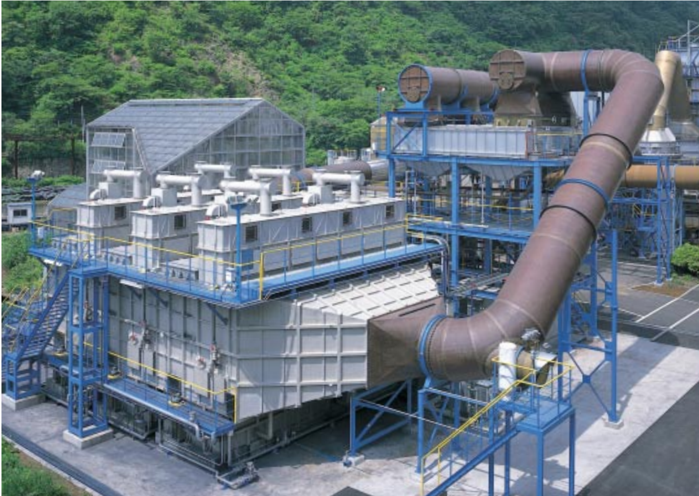
Incineration Plant, Hitachi Works
